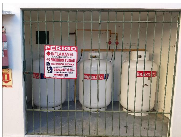
Figura 11 – Central de GLP.
